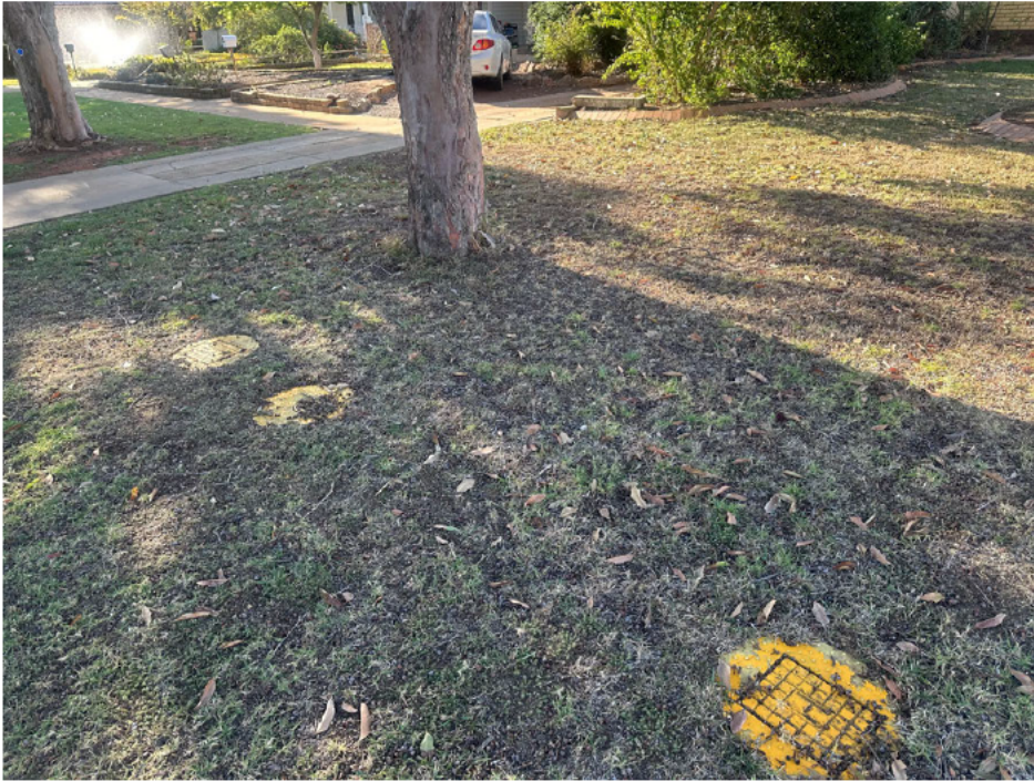
3 x stop valves and hydrants in nature strip
