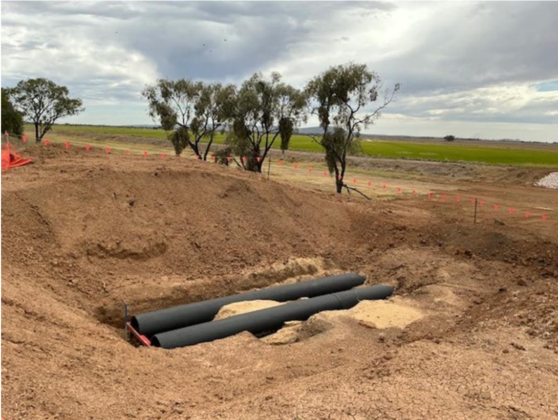
Photo of the pipes from the Main Canal for the North Merribee Channel Realignment. Photo taken 28 th February 2025.
