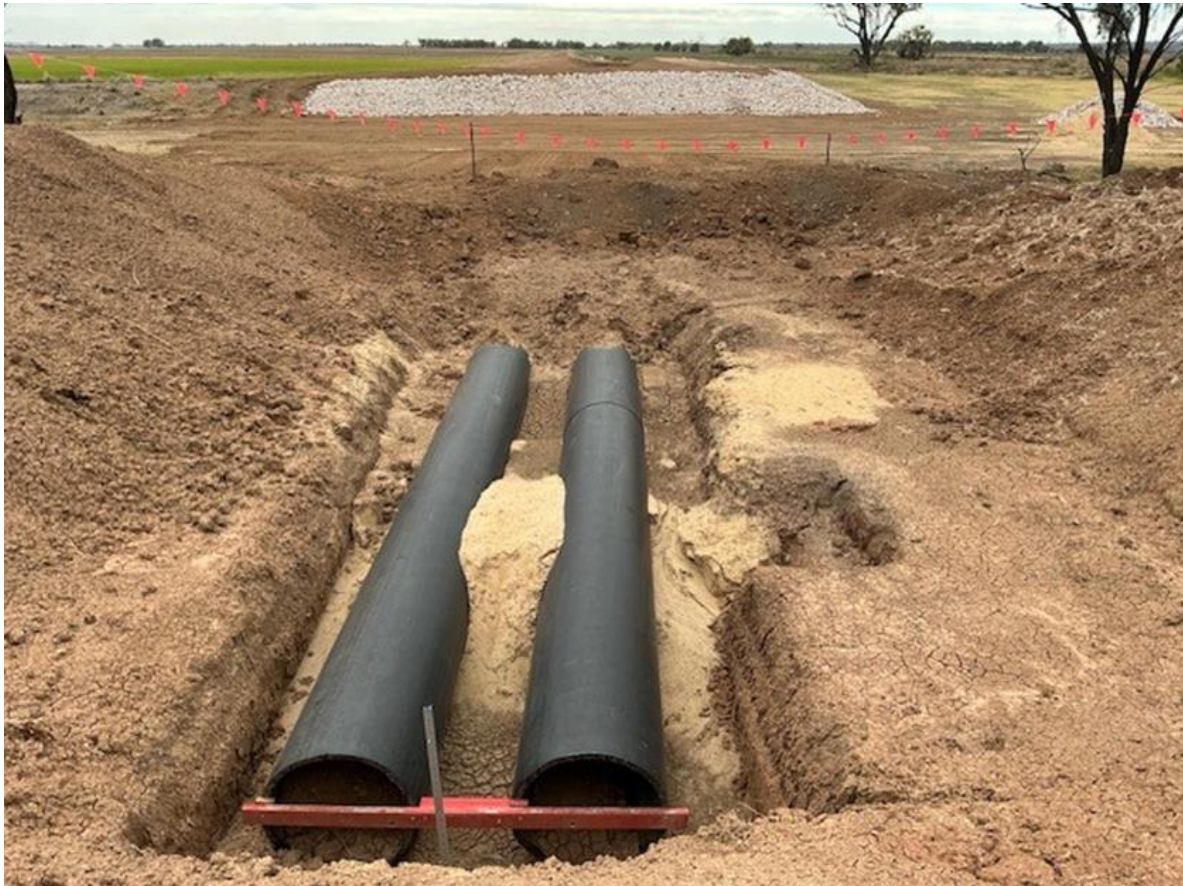
Photo of the pipes from the Main Canal for the North Meribee Channel Realignment. Photo taken 28 th February 2025.
